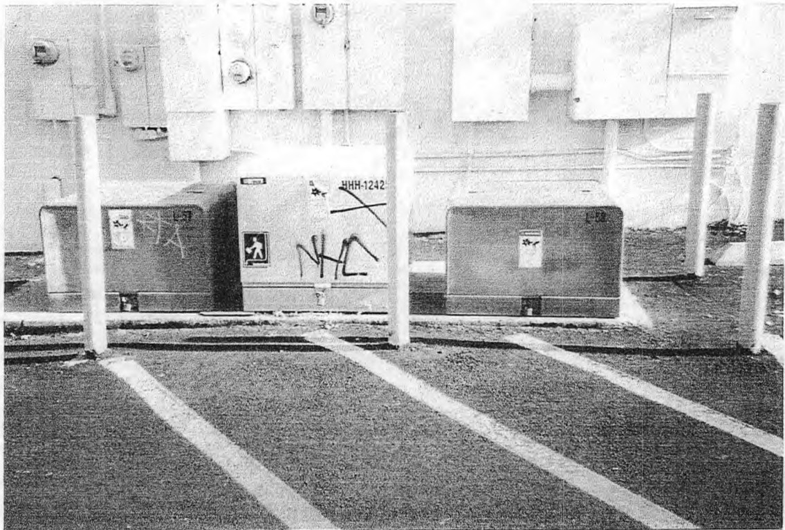
Photo #8: Typical pad mounted transformers located at the subject property. These units are sitting off the northwest corner of building facing Industrial Rd.
