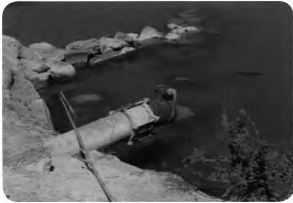
Pump backflow pipe. The pump system which replenishes the lakes from on site wells backflows into Tule Springs Lake. The irrigation system is supplied by the Lakes. The Park full-time maintenance staff are responsible for maintaining the pumps and irrigation system among other duties.
