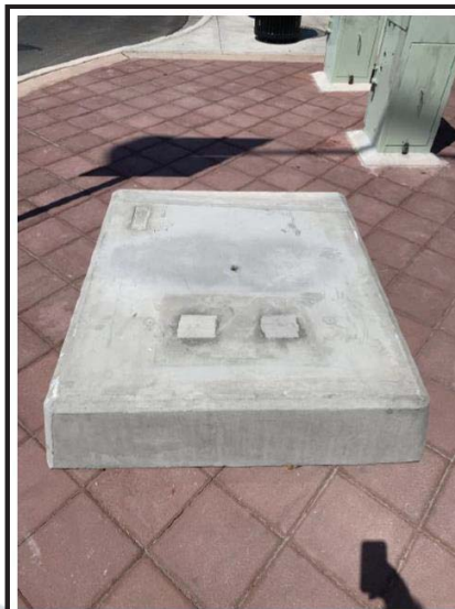
Pedestal #1 - Main St. & Colorado (NE Corner)
