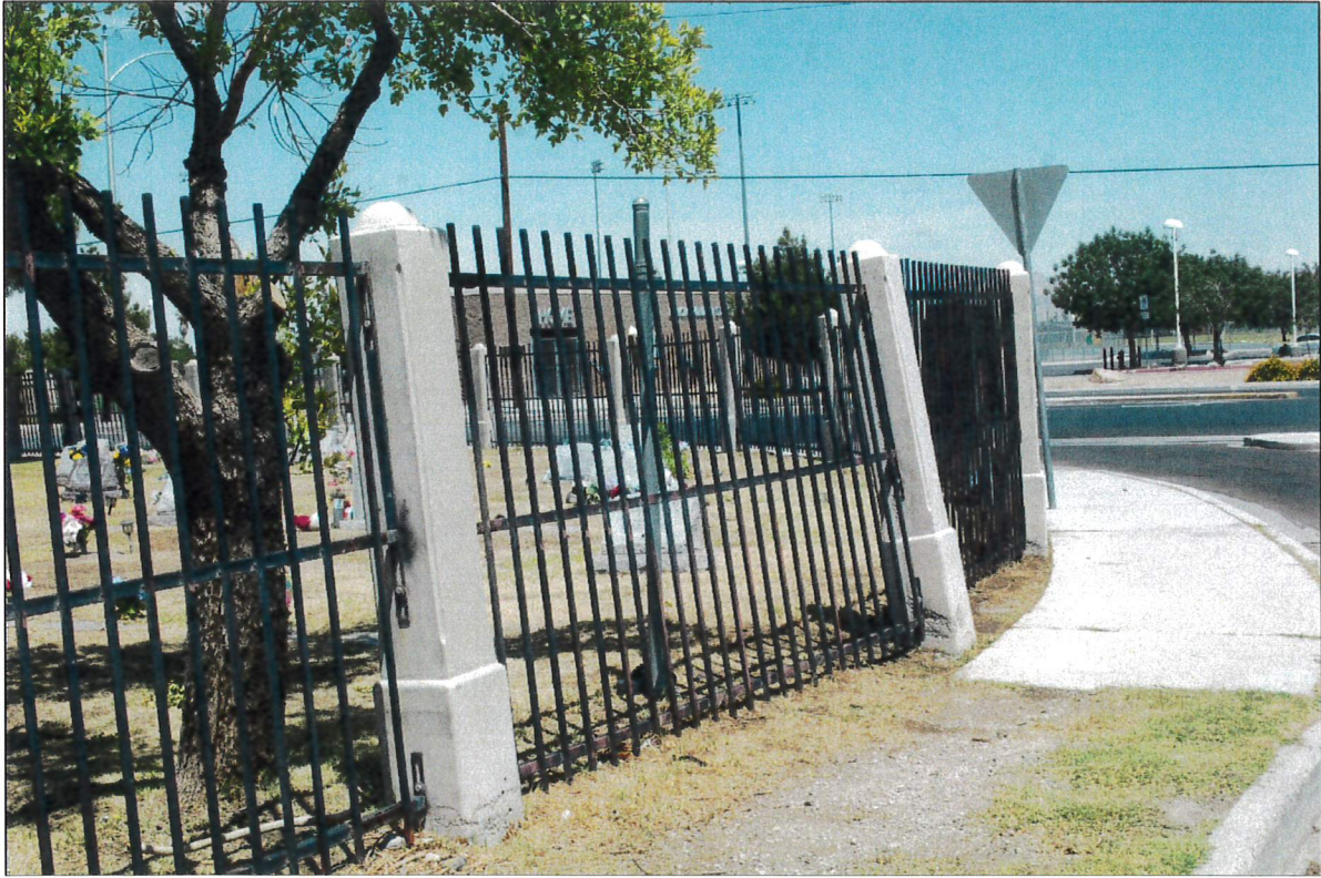
Image 6: Damaged and bowed fence.
