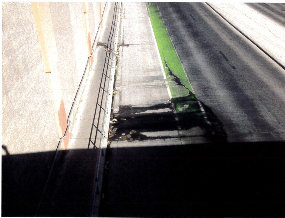
Figure 3 Groundwater Seepage from the Bonneville Avenue Underpass
