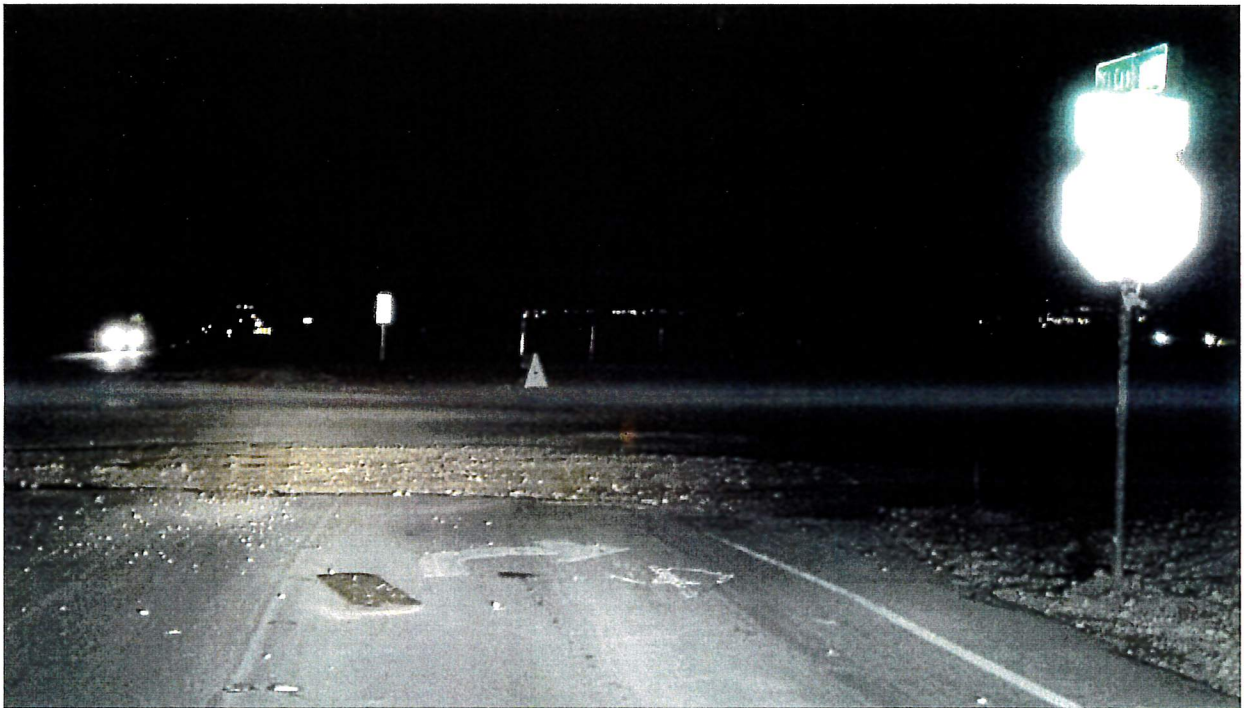
EL CAPITAN / ANN ROAD – FACING SOUTH (8/22/2016 STORM EVENT) SEDIMENTATION ALONG NORTH AND SOUTH HALF OF ANN ROAD, WEST TO EAST
