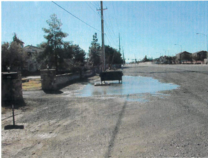
Standing Water at Low Spot in Roadway
