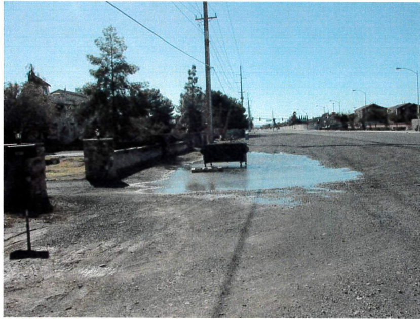
Standing Water at Low Spot in Roadway
