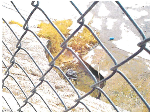
Las Vegas Wash at Carey Avenue looking at lining failure on south side.
