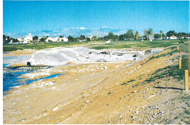
Las Vegas Wash and Flamingo Wash confluence after lining failure shortly after installation.
