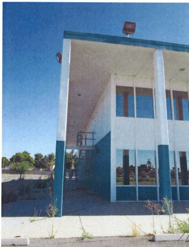
SW corner of South façade. (Area of extensive fire damage in 1992).
