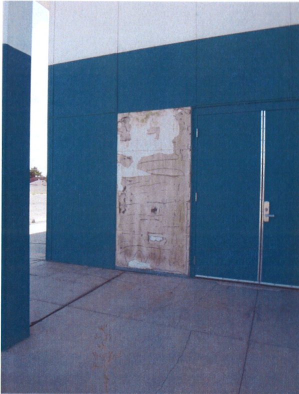
Missing panel on West façade on South corner.
