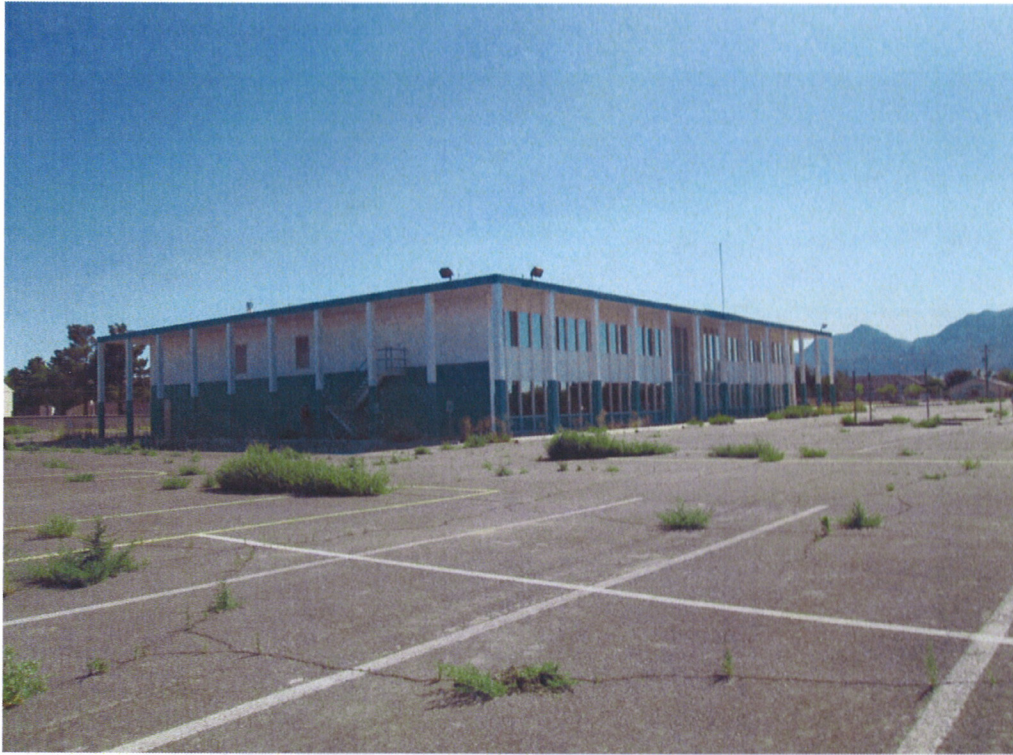
View of SW cornder of building. (The most extensive damage from the 1992 fire occurred here).
