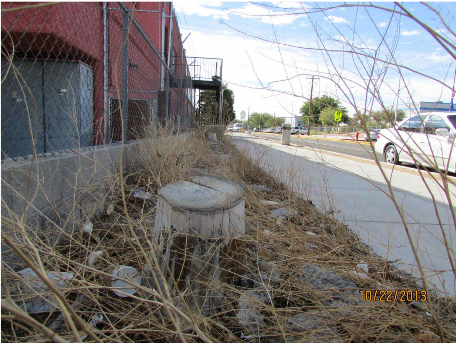
West side of building along back street facing Hyde Middle School. Dead weeds, trash and two large tree stumps.
