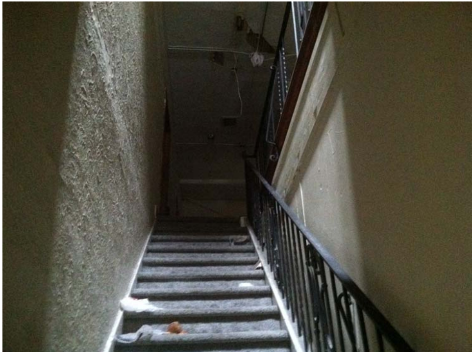
Photograph 8: View of the stairwell with heavy texture.
