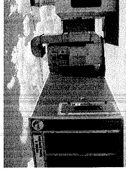
BUILDING 'D' SPRAY BOOTH
