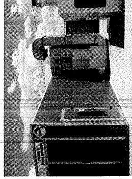
BUILDING 'D' SPRAY BOOTH
