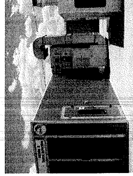
BUILDING 'D' SPRAY BOOTH
