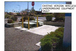
VIEW OF EXISTING VZW EQUIPMENT VAULT (LOOKING NORTHEAST)
