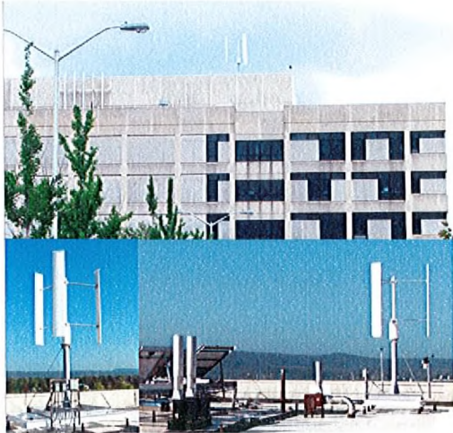
Roof-mounted vertical axis system Manufacturer: Cleanfield Energy Location: Blacksburg, Virginia
