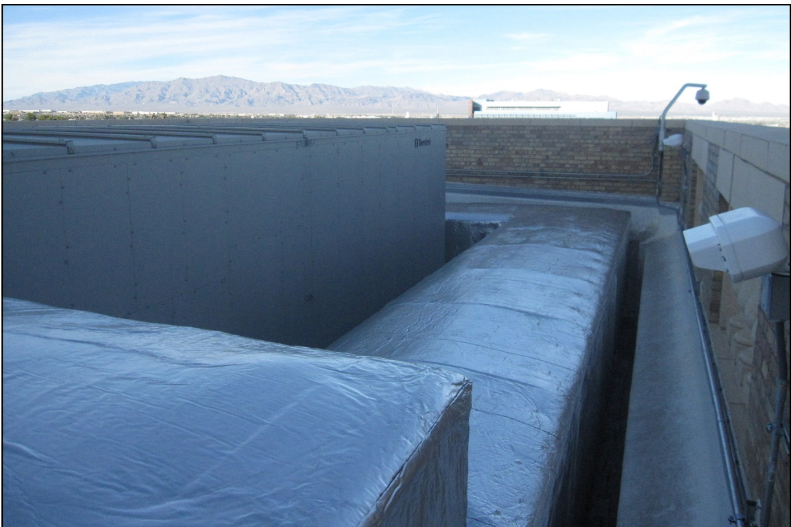
Photograph 84: Air handlers and ductwork, view northwest
