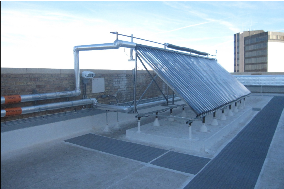
Photograph 82: Solar equipment at roof, view northeast
