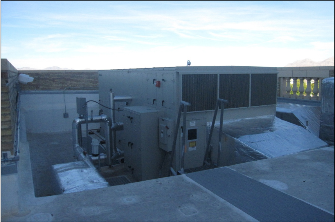
Photograph 83: Air handlers and ductwork, view northeast
