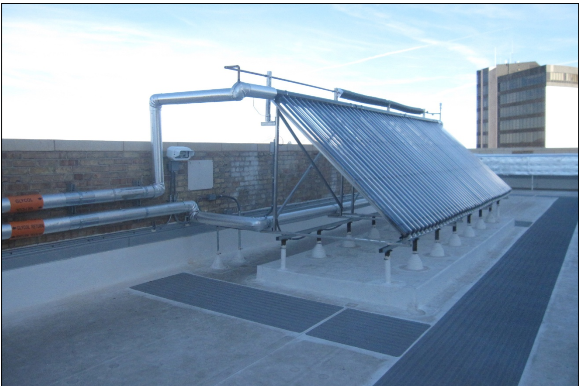
Photograph 82: Solar equipment at roof, view northeast
