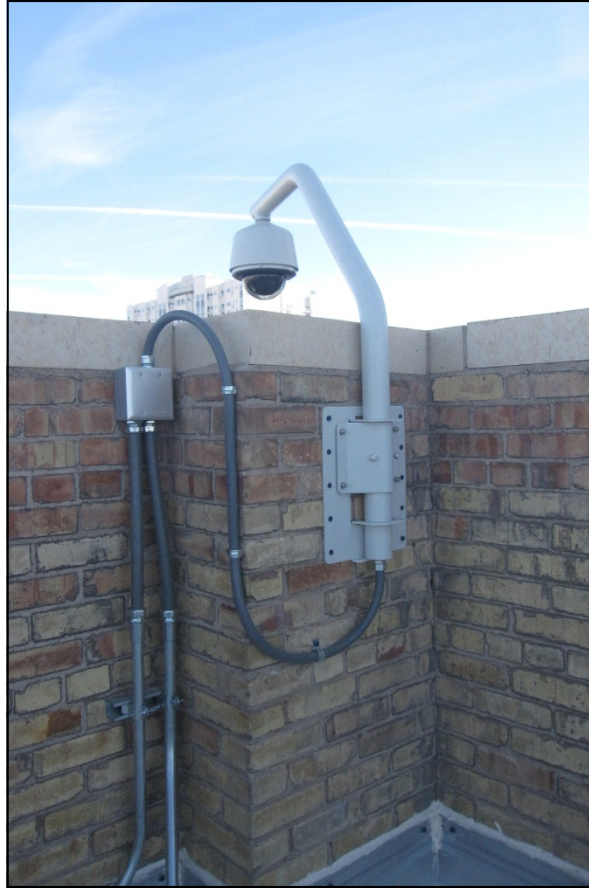
Photograph 85: Security camera, view southeast, note typical
