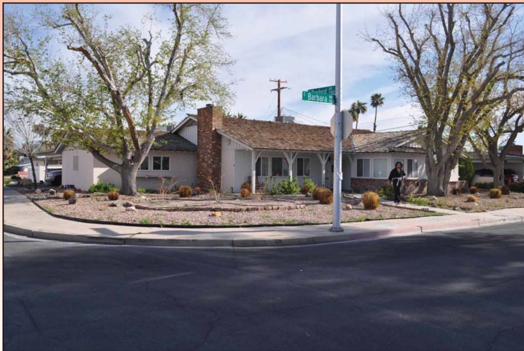
Figure 4.10 A shake roof at 545 Barbara Way.
