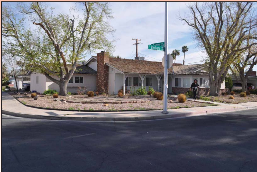
Figure 4.10 A shake roof at 545 Barbara Way.
