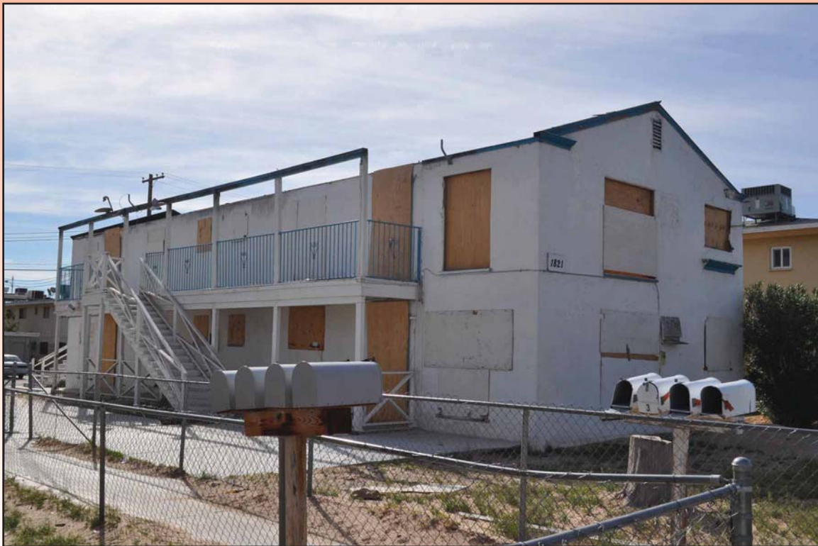
Figure 3.54 Deteriorating condition evident on this four-plex at 1821 Santa Paula Drive.
