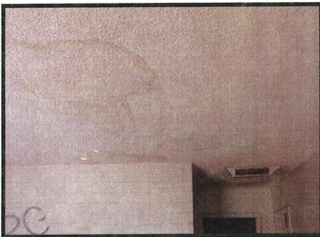
Unit A – Ceiling Damage
