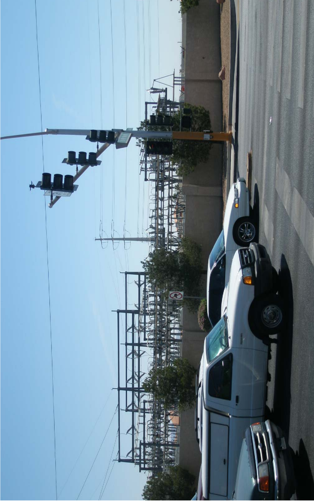
SUP-30324 - APPLICANT/OWNER: NEVADA POWER COMPANY NORTHEAST CORNER OF CHEYENNE AVENUE AND DURANGO DRIVE OCTOBER 23, 2008 PLANNING COMMISSION
