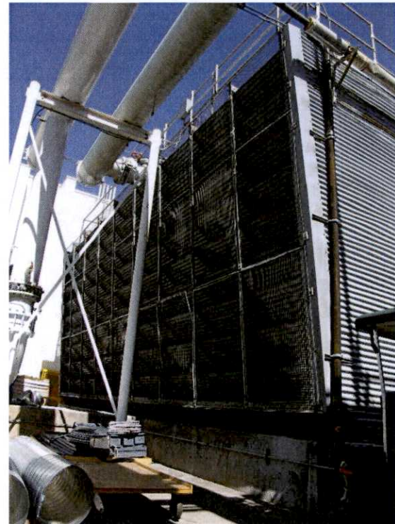
Image: Commercial cooling tower
