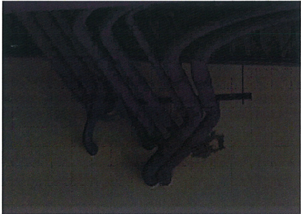
COAX SHELTER ENTRY PORT
