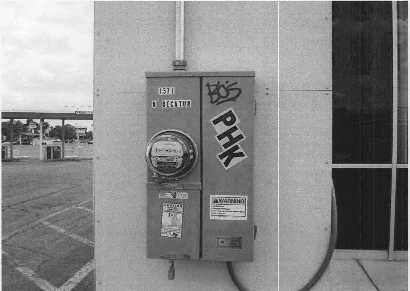
Graffiti noted on power meter of subject billboard.
