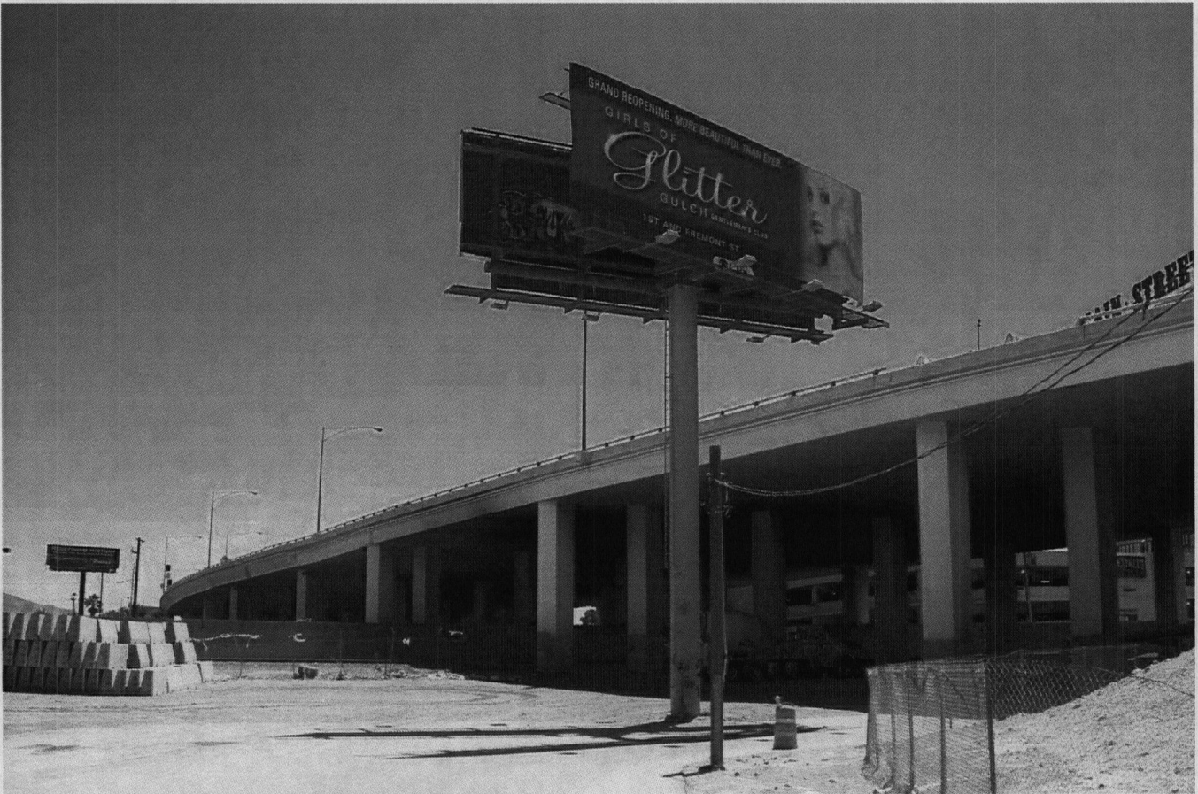
West façade of billboard, note graffiti at base of pole.
